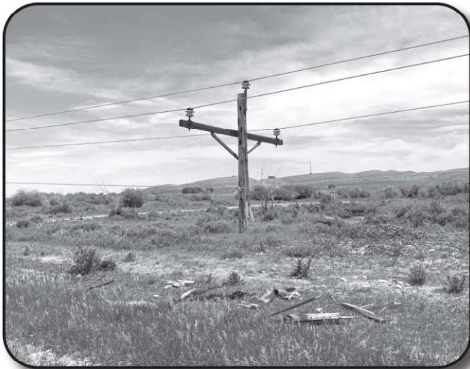
Vehicle vs power pole between Ethete and Ft. Washakie.
