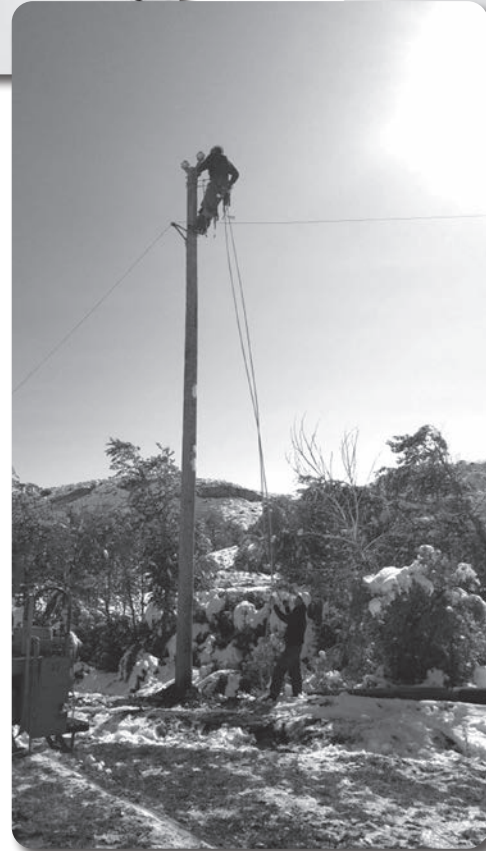
LINE FOREMAN BRIAN HEINER AND APPRENTICE LINEMAN KYLE CARPER WORKING TO REPAIR THE BROKEN POLE SHOWN IN THE PHOTO ABOVE
